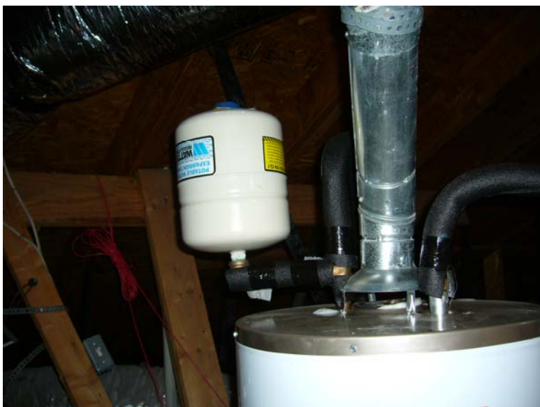
4 example of an expansion tank file photo
