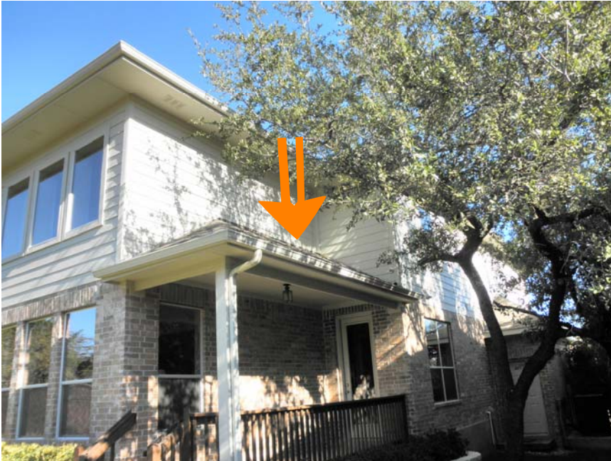
1 trees close to roof and no air vent on roof over patio
