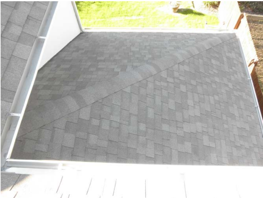
2 no air vent on roof over MBR
