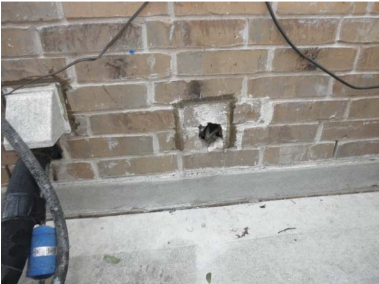
3 hole in brick on left side of home
