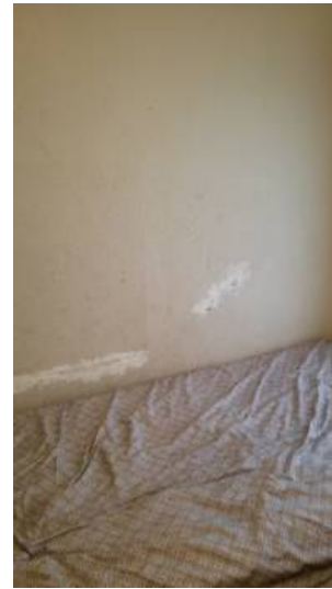
damaged sheetrock left front bedroom.
