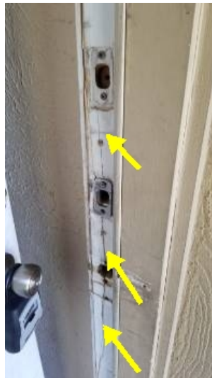
Front door jamb is damaged at the striker plate area.
