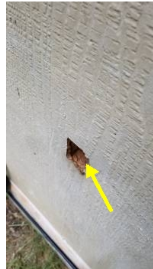
hole in the siding on the right side of the house
