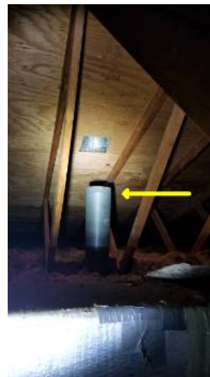
range hood vent pipe terminates in attic.
