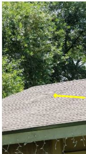
roof decking damage on the front left corner of the house
