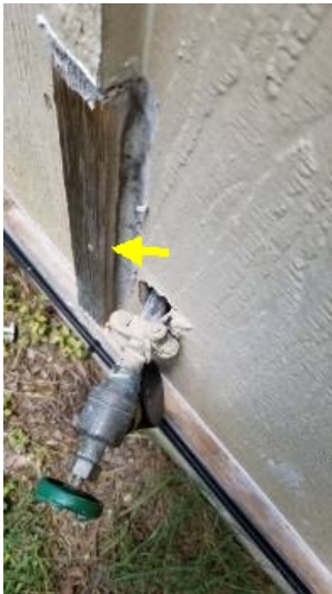
damage wall trim
