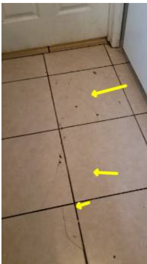
kitchen floor tiles cracked.
