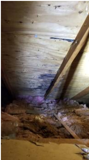
Roof wood decking shows signs of water damage on the front side.
