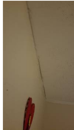
garage ceiling sheetrock sagging.
