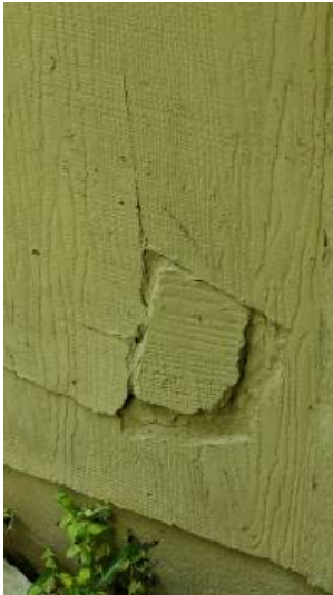
damaged siding on the left side of the house
