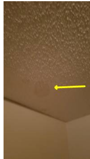
water stain on ceiling sheetrock.
