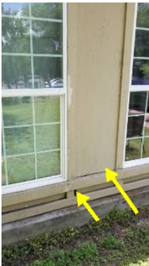
siding and trim damaged front side.
