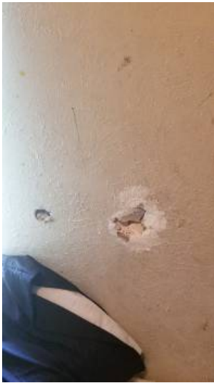
damaged sheetrock left front bedroom
