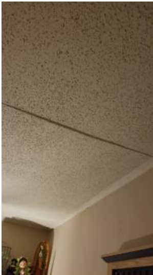
converted garage ceiling sheetrock sagging.
