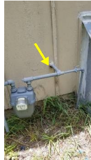
Gas lines are not bonded to electrical panel. Wasn't required when house was built.
