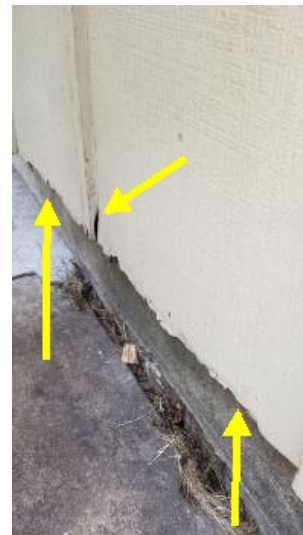
siding and trim damaged left side of converted garage.
