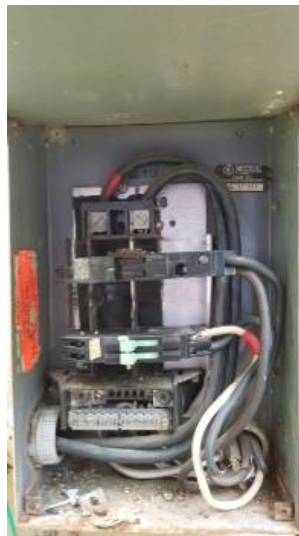
Both electrical panel boxes are zinco brand. These electrical panel boxes are considered a safety hazard. Recommend replacing electrical panel boxes.
