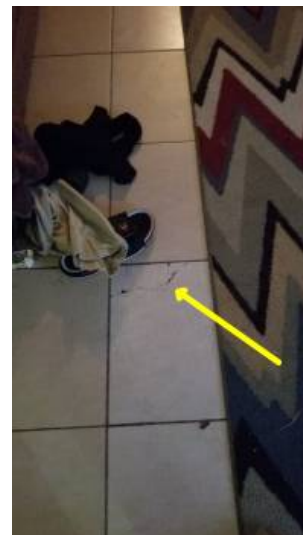
living room floor tiles crack
