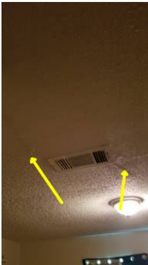
ceiling sheetrock cracked and sagging
