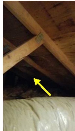
Roof wood decking shows signs of water damage on the front side.
